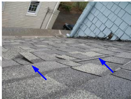
Lifting shingles/slipping shingles
