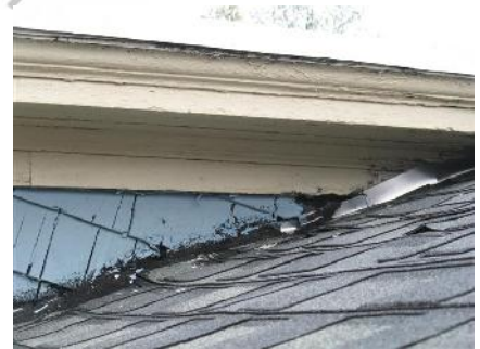
Poor quality flashing installation
