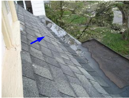
Slipping shingles, gutters holding water
